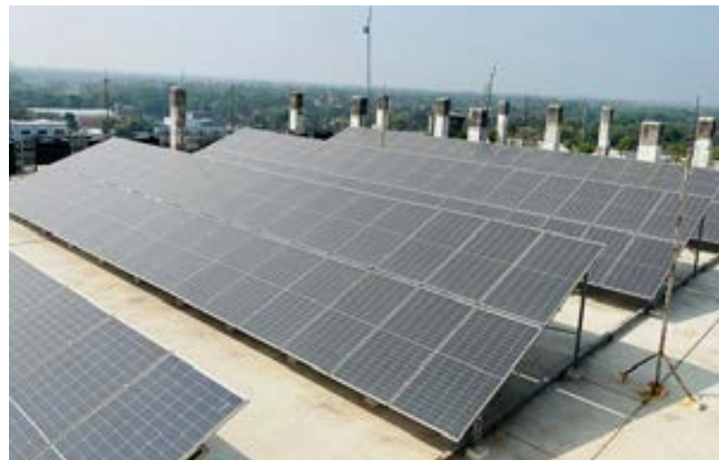
Figure 2: The factory has a rooftop solar system with a capacity of 67kW.
